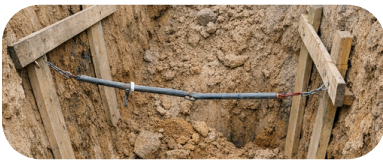
Trapped in a Trench Collapse
