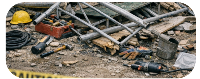
Pinned by Collapsed Scaffolding
